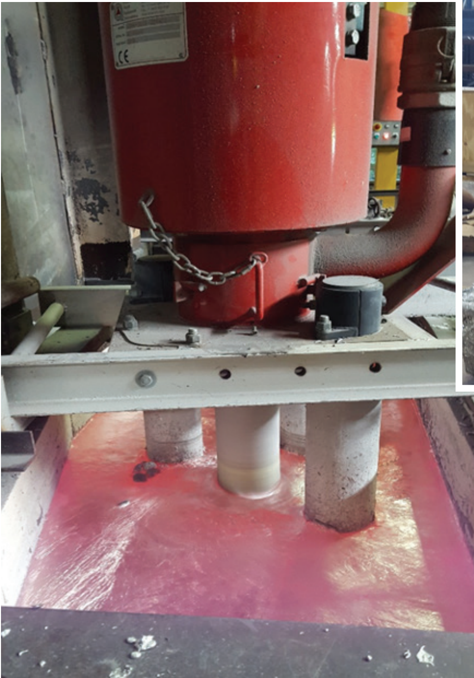
Clean well after 4 years of routine cleanings
